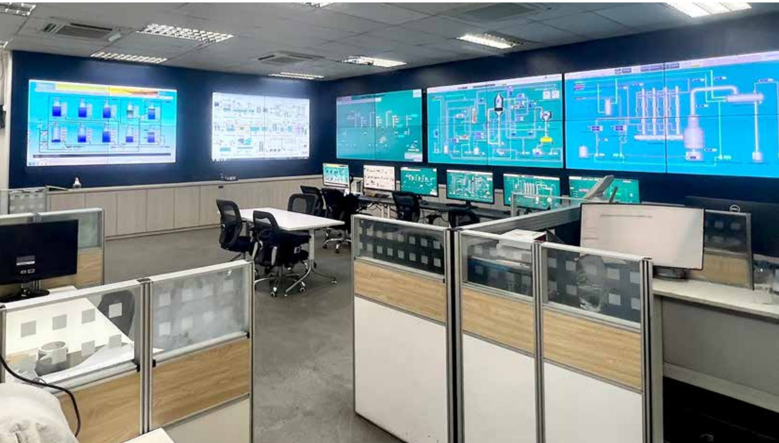
Operation Control Room
