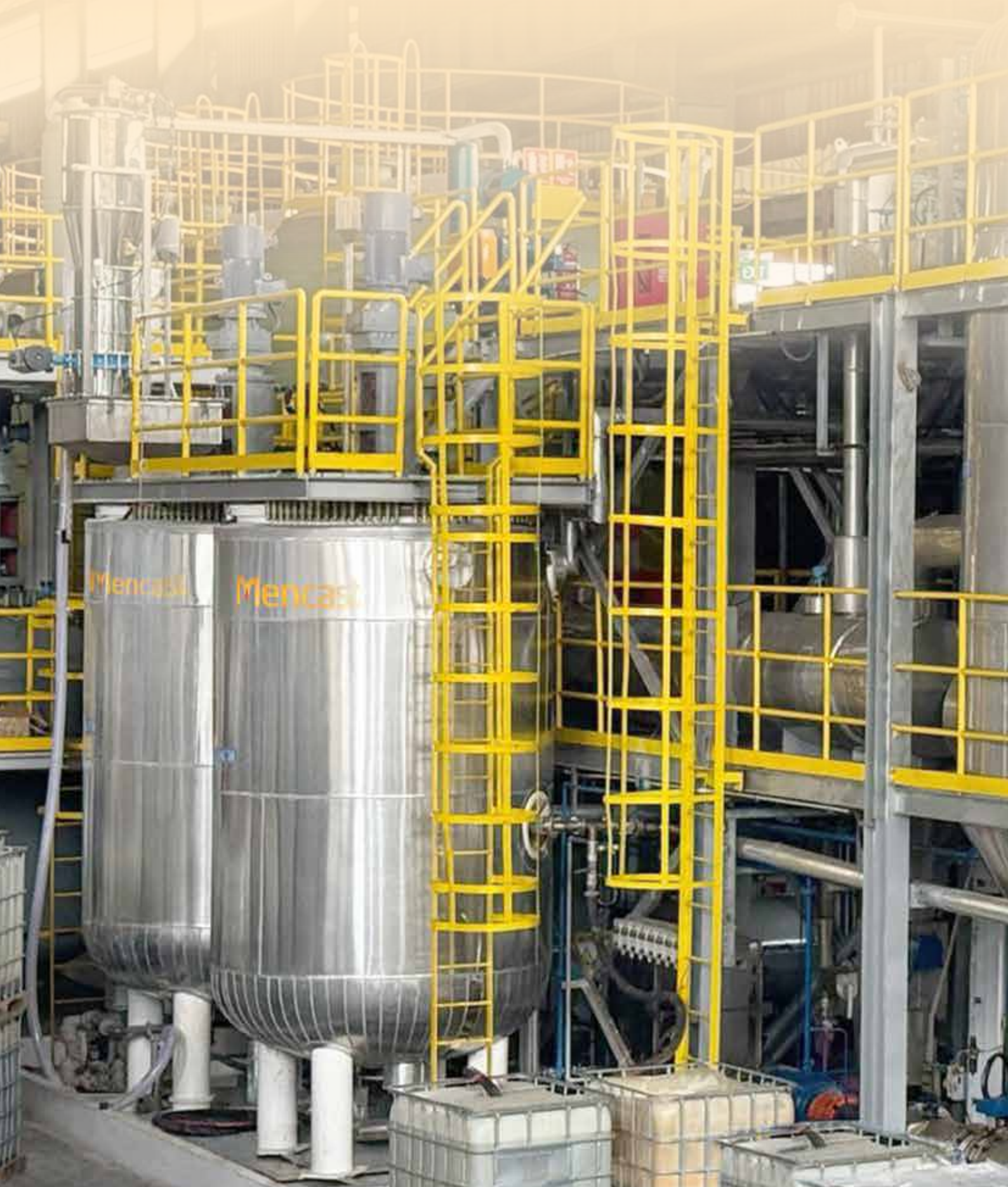
Advanced treatment plant recovers useful byproducts from sodium hydrosulfide (spent caustic), enabling circular sustainability
