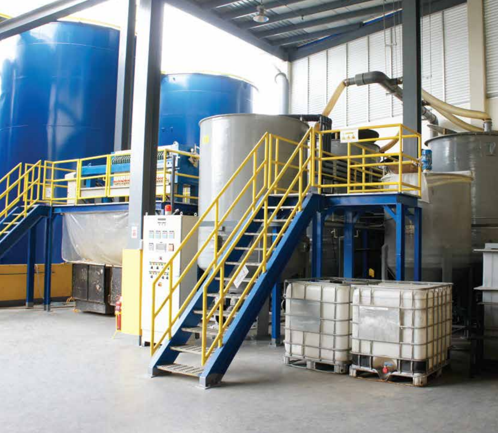
Waste Water Treatment Plant
